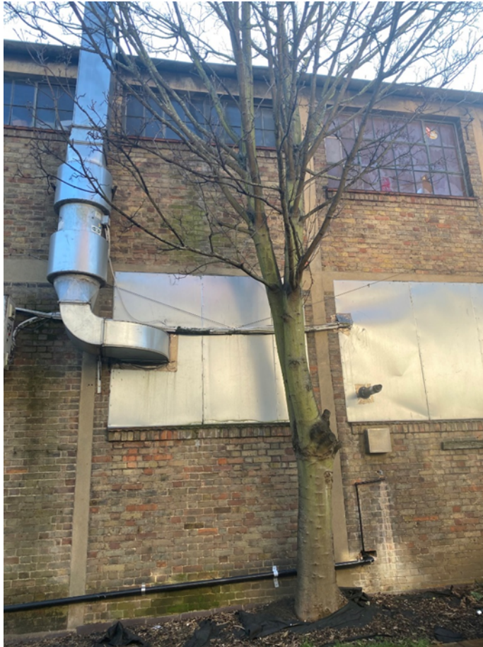
Figure 12 North Flank of Existing Building from the Rear Garden of 1A Brassie Avenue
